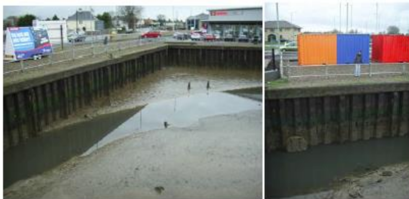
Plate 5-2 - Sheet pile wall in Lowestoft acting as informal flood defence (extract from SFRA)
